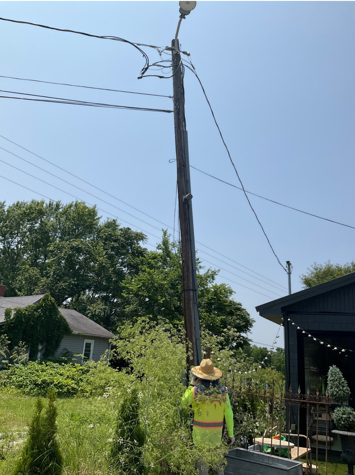
Communications attachments are above the top of the electric service riser in the power space.
